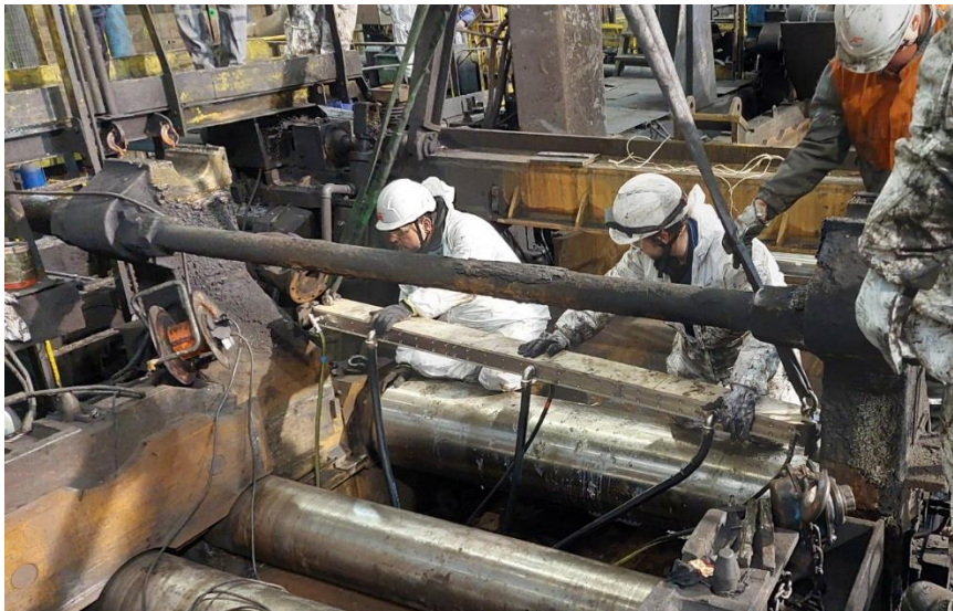
Figure 7 – Mechanical installation on the hot rolling line with all electrical and cooling cables connected.
