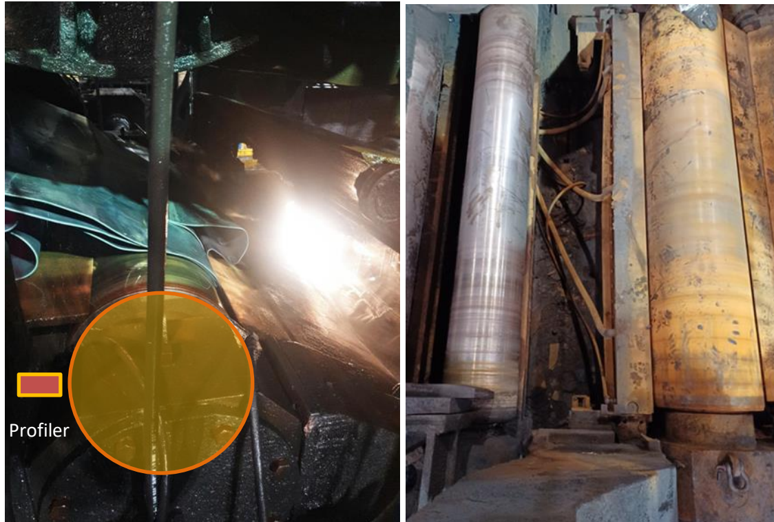
Figure 4 – View of the coiler & Roll Profiler after the major incident
